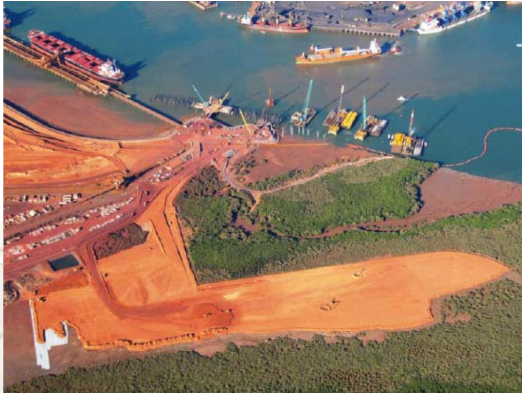
The new Utah Point berth and stockyard under construction at Port Hedland showing the existing No. 1 berth and manganese loader in the background
