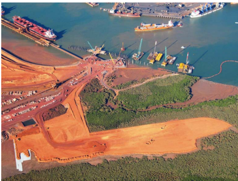
The new Utah Point berth and stockyard under construction at Port Hedland showing the existing No.1 berth and manganese loader in the background. The new berth, stockyard and loader are currently scheduled for completion towards the end of the third quarter of 2009.
